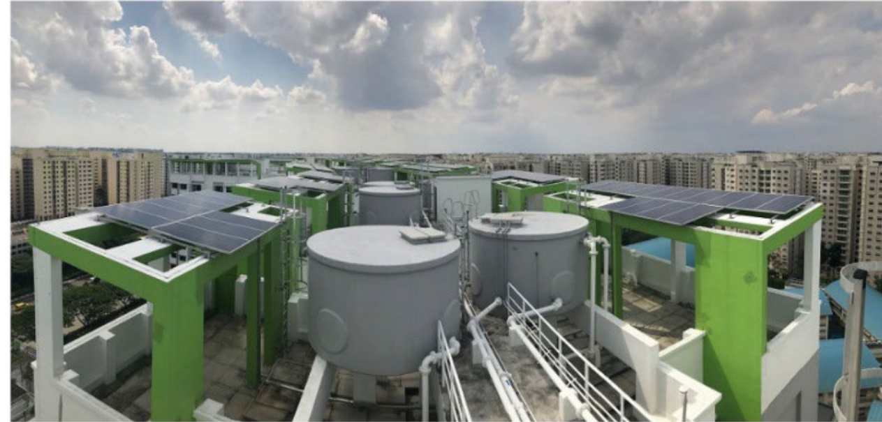
Essential block services such as water tanks and lift motor rooms were strategically located to optimise available space for installation of solar panels on the roofs, with access routes planned for easy maintenance
